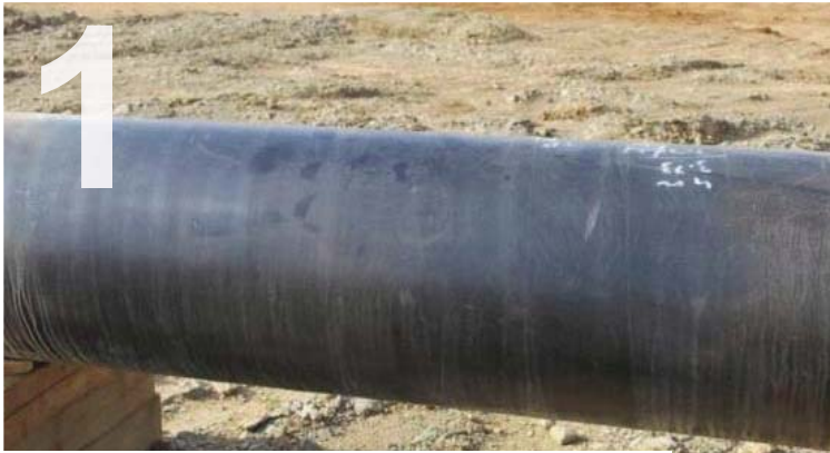
2m circumference PVC coated multi-purpose fuel/oil pipeline
